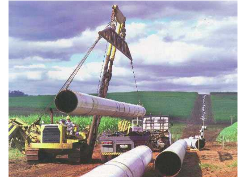
High Strength Steels for Natural Gas Pipelines
